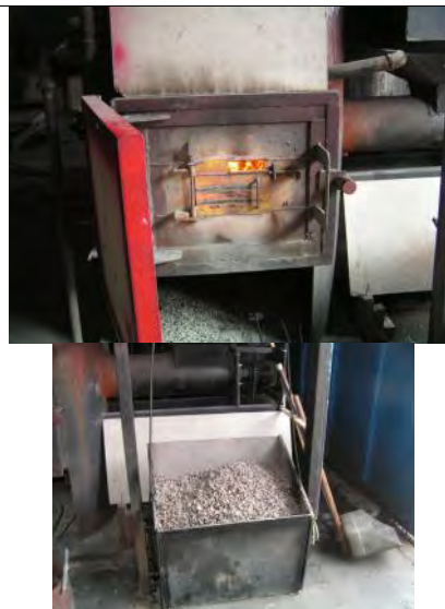
Photo 44) Boiler section ( Waste of Palm shells)
