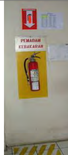
Photo 40) Sample Fire extinguisher
