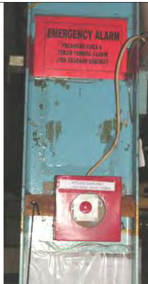
Photo 41 ) Sample Fire Alarm
